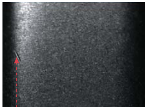
Normally, the dent in this image could not be detected because of the random glare and granular texture of the metal.
